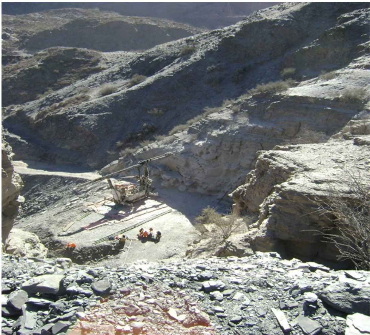
Installing grouted steel pipes at a tunnel portal for pre support of initial excavation rounds.
